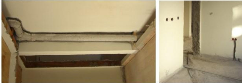
Figure 24. Waste water piping and heating system and power socket
